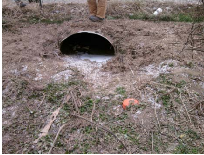
Surface riser nearly buried by sediment and debris near roadside culvert.
